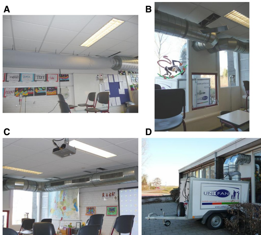
Figure 1 Installation of the ventilation intervention in a classroom. A = air sock for air supply, B = tailor made window pane, C = non-flexible duct for air exhaust, D = ventilator.
